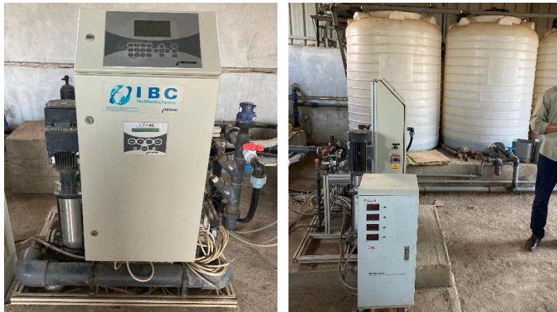
Fig. 33 & 34 Automated fertigation system at a nursery
