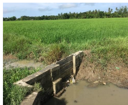
Figure 2 Small sluice gate in Kungyangon
