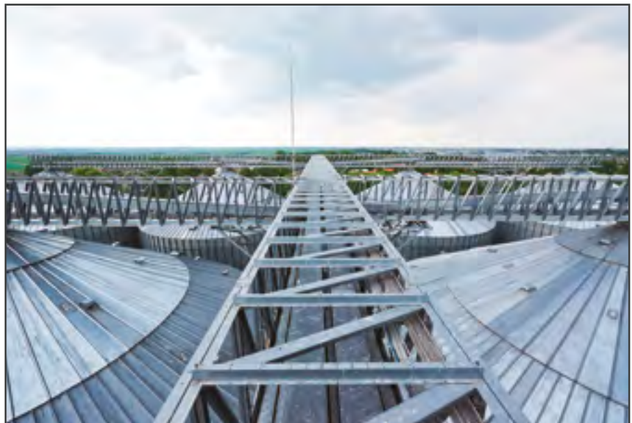
Grain silos in southwestern Ukraine (Mriya)
